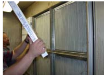
Specified Filters Prior to Test
