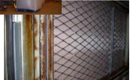
Leaks through Washables
